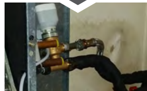
Upgraded/replaced valves and pipe insulation reduce risk of breakdown and condensation damage.
