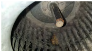
Dirty Fan Blades cause vibration and reduce the fan bearing lifetime.
